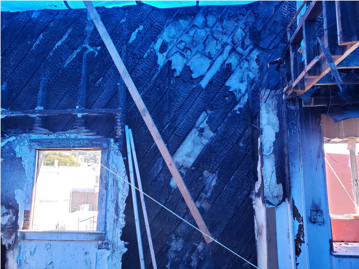
2 nd Floor stud walls have been destroyed. There's no gravity or lateral support for the walls.
