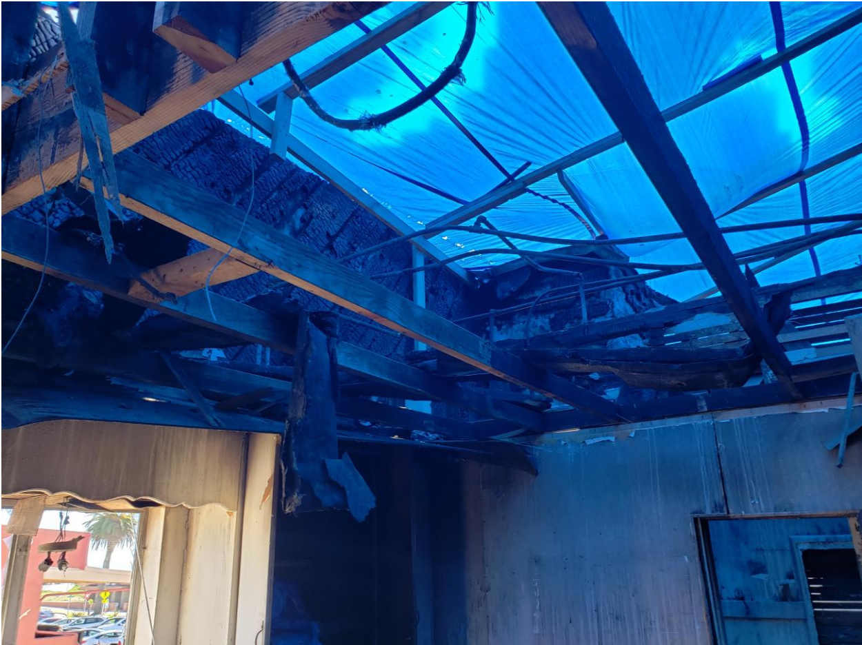
The roof have been completely destroyed by the fire. There's no lateral support for the walls.
