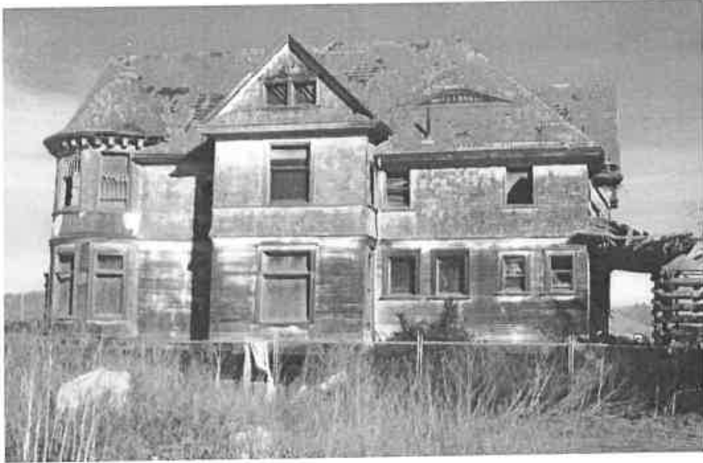
Photo #3. Looking East at the West side-elev., note condition of building fabric, missing features & fenestration, Kent Seavey, December 29, 2024.
