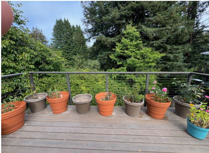
④ VIEW TOWARD PROPERTY LINE – CORNER OF DECK ENCROACHES INTO SETBACK
