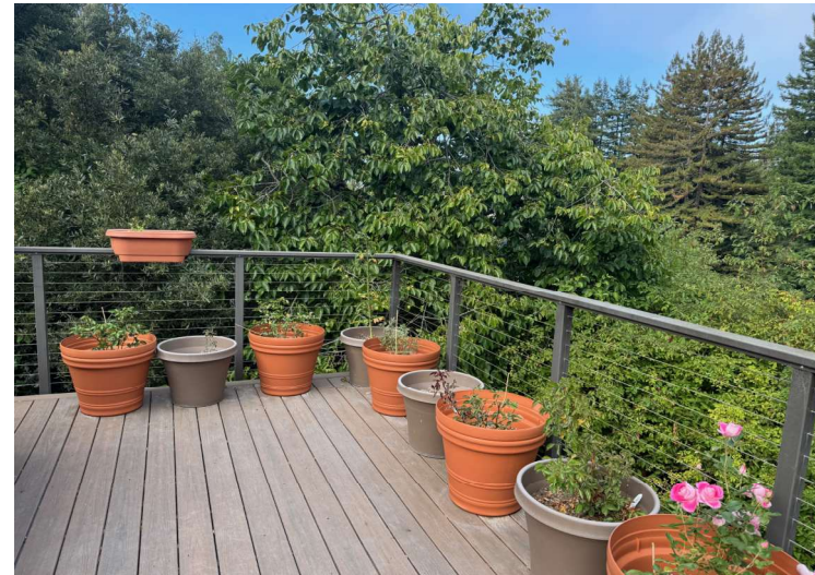
② VIEW TOWARD PROPERTY LINE – CORNER OF DECK ENCROACHES INTO SETBACK
